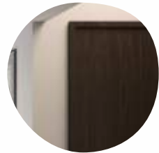
Flush doors with sal wood frame
